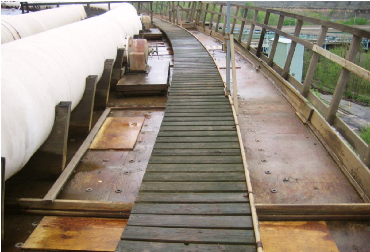
Wood Crossflow Cooling Tower Prior to Reconstruction
