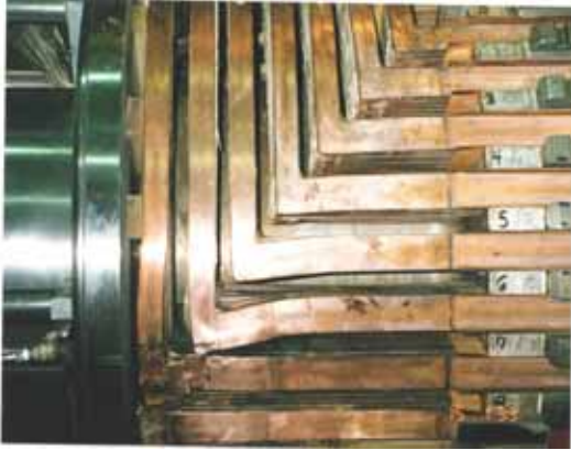
Figure 1: End-strap elongation has distorted the top turn of the #6 coil resulting in contact with the top turn of the #7 coil.
