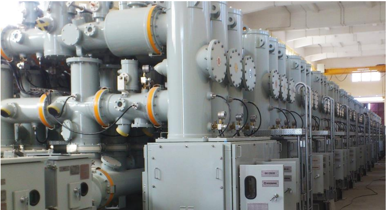
Figure 3: GIS with arc detection system
