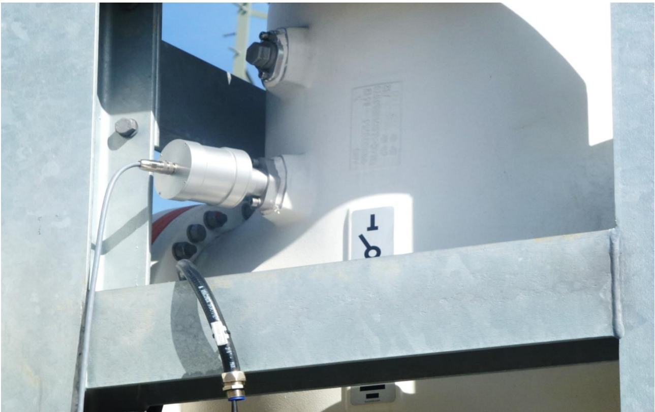
Figure 13: OTEM on 400kV disconnector/earthing device
