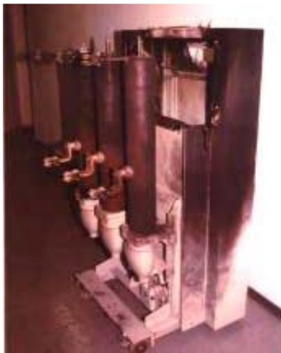
Figure 11: Shutdown without arc detection and phase error system
