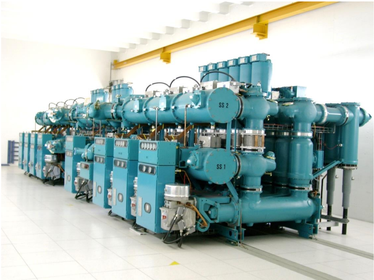
Figure 2: GIS with arc detection system
