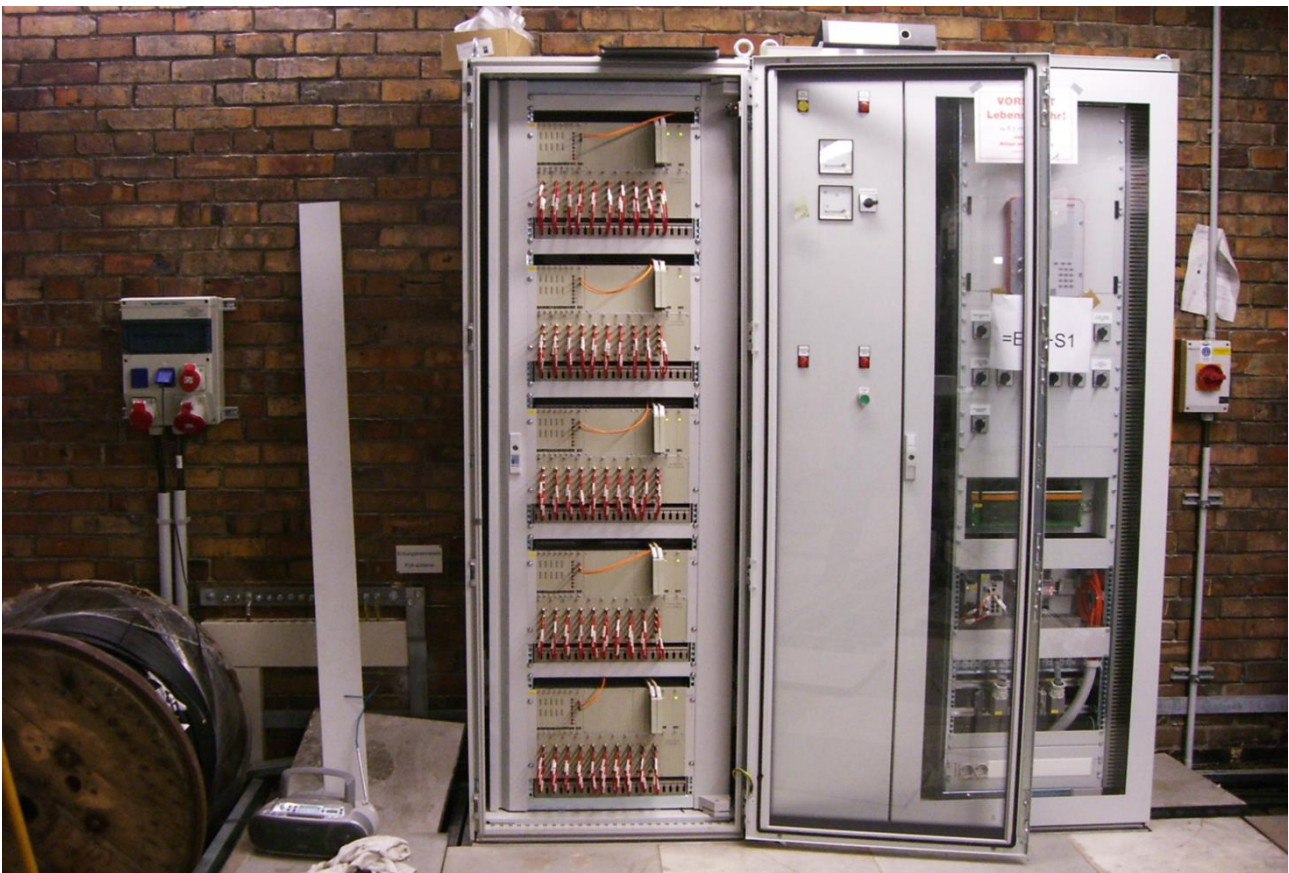
Figure 6: Control cabinet with LIBO devices
